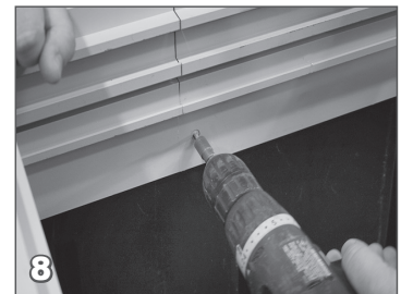
8 Secure the riser to the housing by screwing 1 inch self-tapping screws (H9614) through the riser and into the housing. Make sure the top of the riser is flush with what will be the finished deck height.
