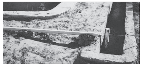
(4.b.) Housing in place mounted on gunite piles ready for deck pour.
